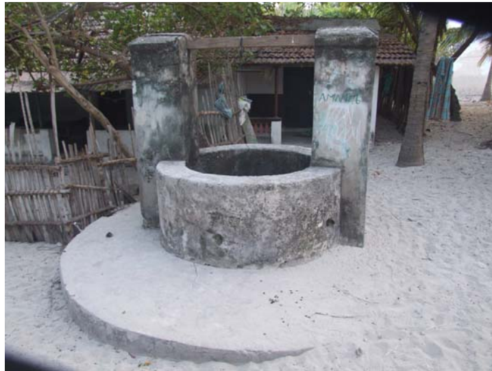
The existing well in Amini Island needs renovation under MGNREGS
